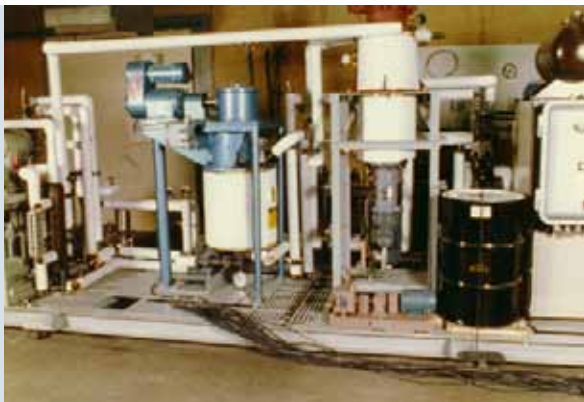
FIGURE 2 – SKID MOUNTED PILOT PLANT
